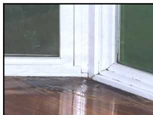
Water Leak = Rotted Wood!
